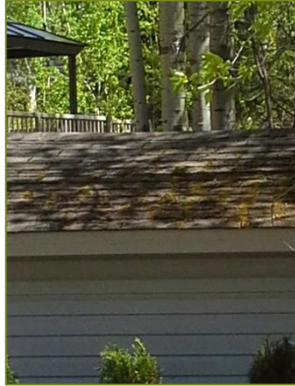
Figure 20. Roof with debris buildup
