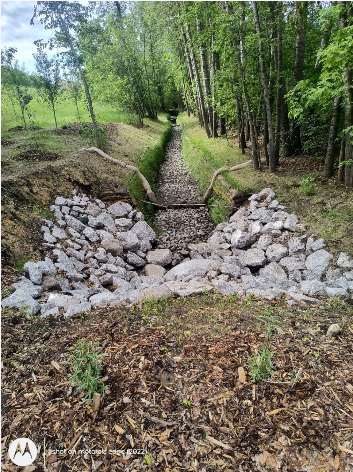
Figure 5 - French Drain Eco Bags (For visualization and example purposes only, depth/width subject to change)
